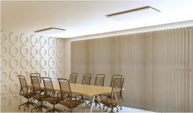
Ceiling mounted MH600UB Infrared heating panel
